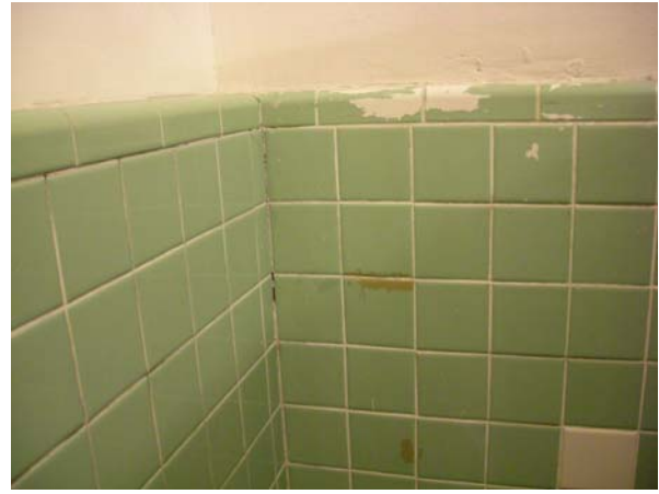
Tile wall damage
