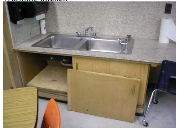
Casework needing replacement
