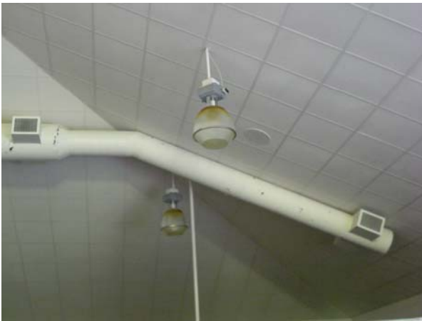
Media Center Ductwork
