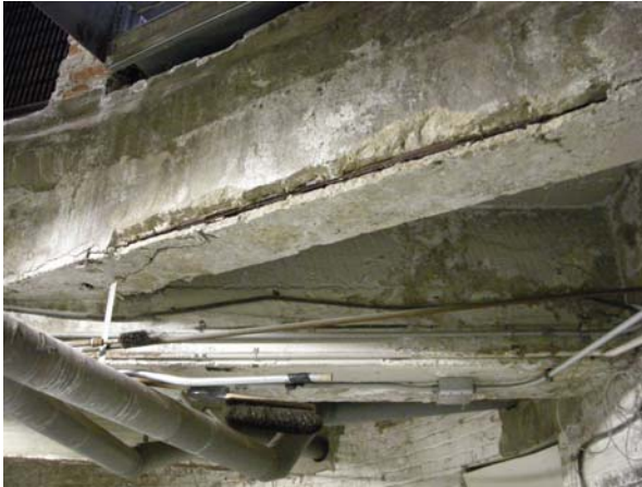
Deteriorating beams in boiler room
