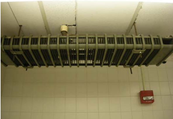
New Radiator in Basement
