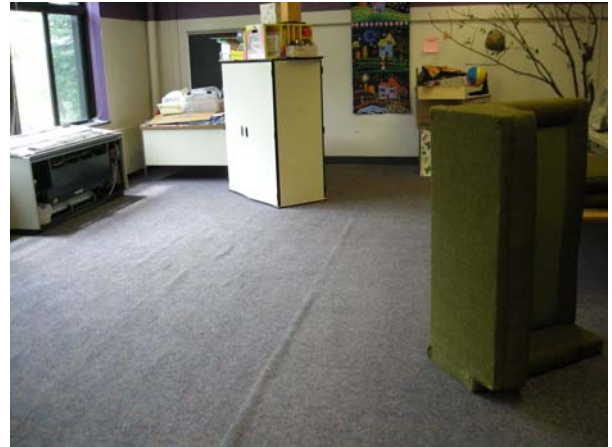
Problematic carpet installation
