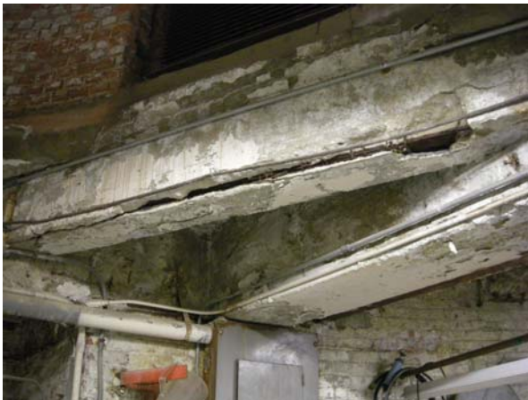
Deteriorating beams in boiler room
