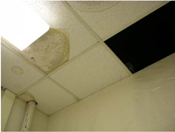
Ceiling water damage
