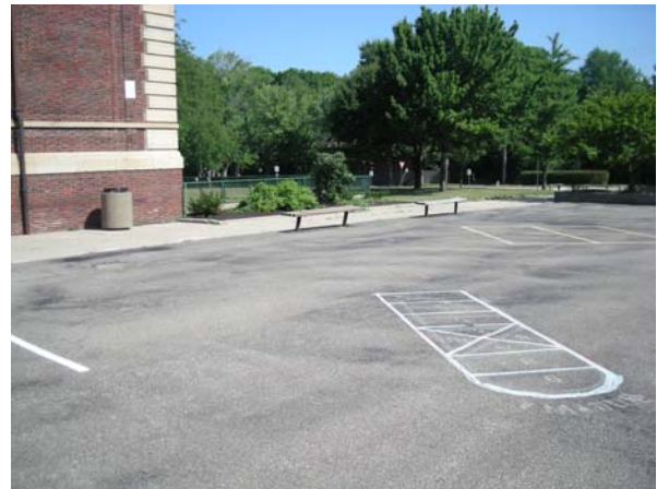
Worn asphalt play surface
