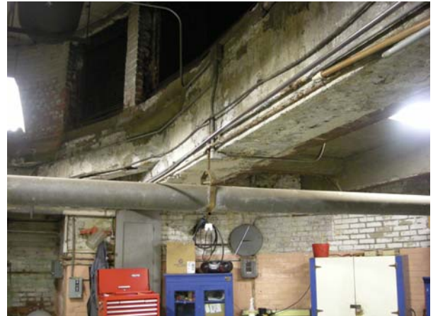
Deteriorating beams in boiler room
