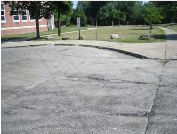
Deteriorating pavement and curbs
