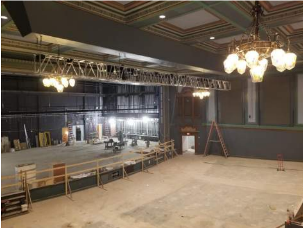
Hanging Auditorium Lighting
